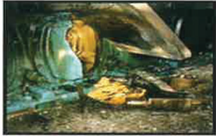
Damaged crankhouse door with broken hinges
